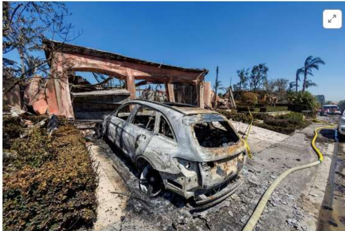
[1/2] A burned car and the remains of a burned-out home are shown after a fast-moving wildfire ripped through an affluent neighborhood in Laguna Niguel, California, U.S., May 12, 2022. REUTERS/Mike Blake/File Photo Acquire Licensing Rights
